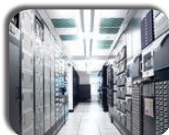
Data Center Management
