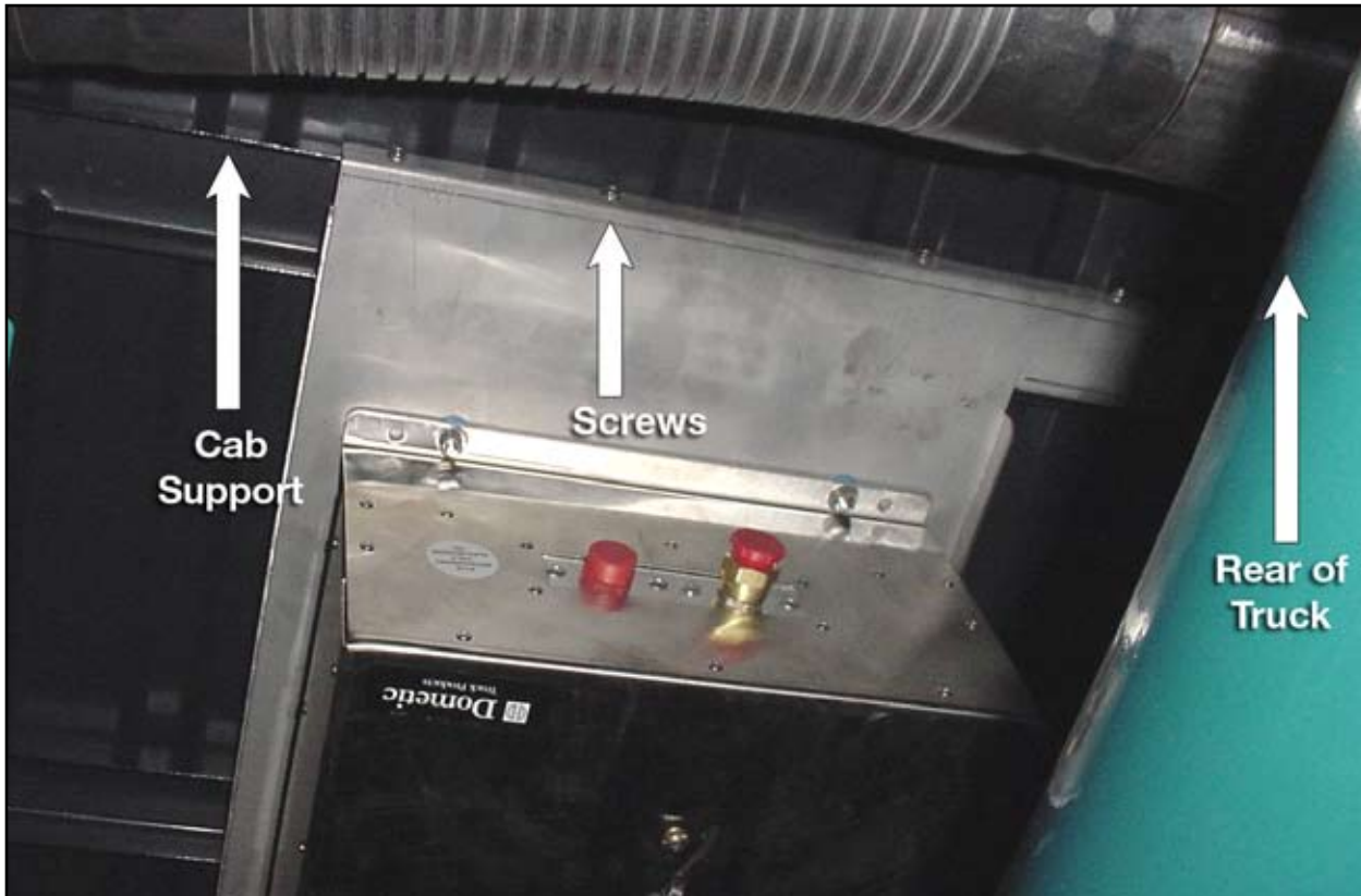
Figure 16. Condenser installed on mounting plate.
