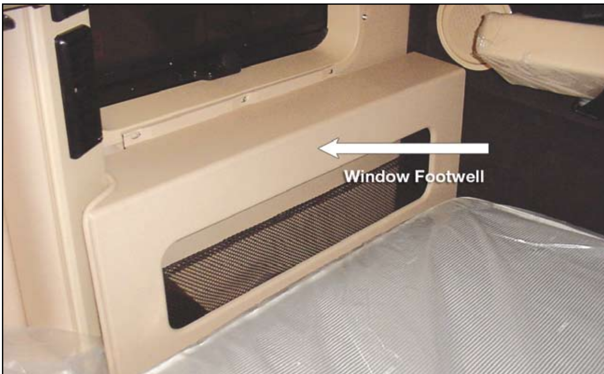
Figure 5. Location of installed ductwork
