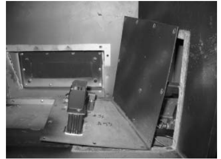
Valve Tray Slightly Removed
