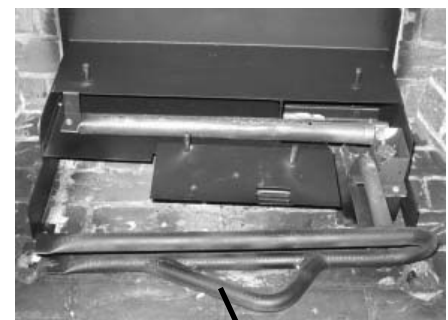
Front Burner Removed
