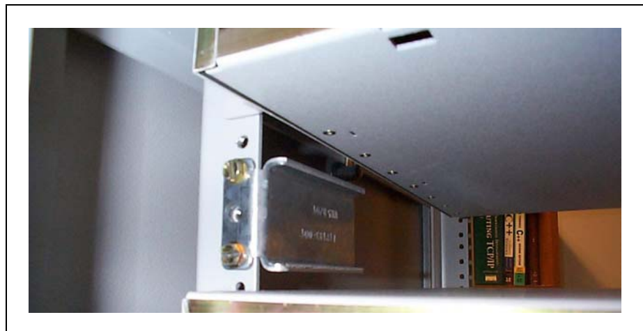
Figure 80 Installed rack-mount bracket
